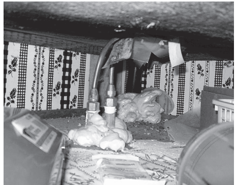
Small leak in cabinet sealed with foam
